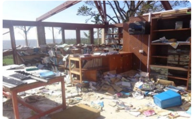
Ratu Kadavulevu School library lost its roof and walls
