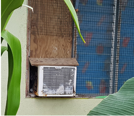
Figure 12: Example of a 'leaky' building envelope and poor efficiency appliance. This window-style air-conditioning unit on Majuro has corroded cooling fins, and is mounted next to louvered window
